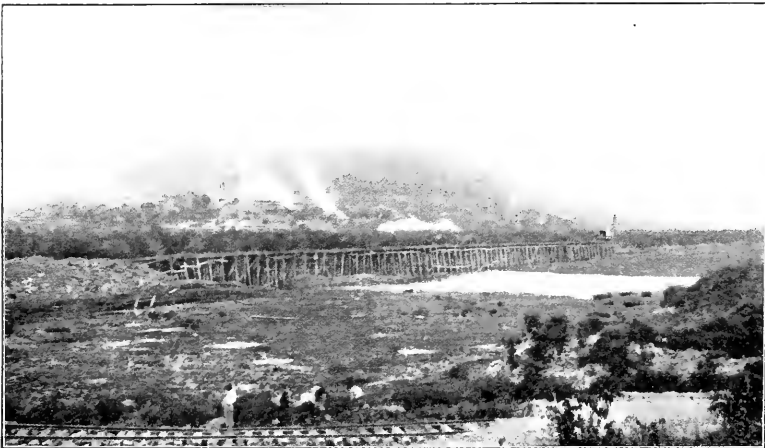
TRISTLE DUMP JUST OUTSIDE OF EAST TOE OF THE SOSA-COROZAL DAM. Ancon Hill and Ancon Hospital buildings in the background.
